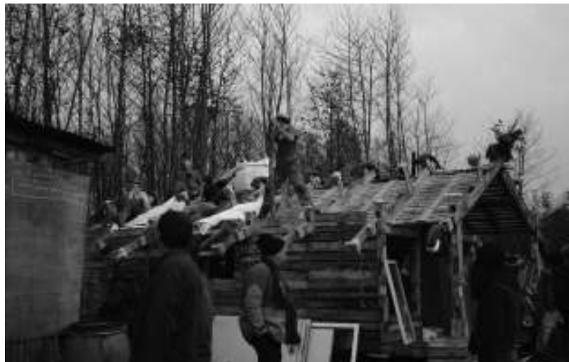
A group works to rebuild some of the infrastructure lost after the 2012 eviction of the ZAD.
