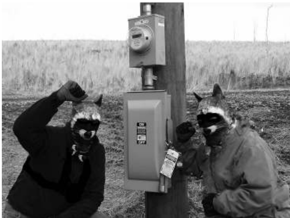
On Christmas Day, anonymous raccoons targeted the Diamond Pipeline in Arkansas, locking the main operating valve to prevent use.
